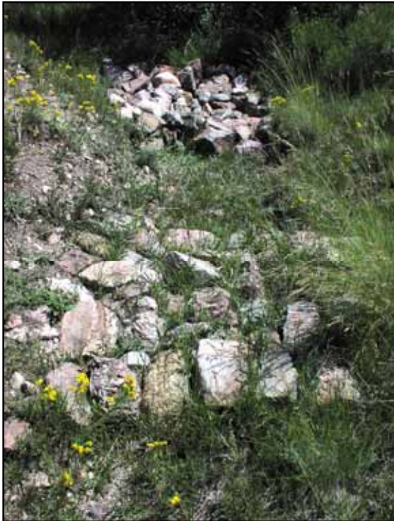
Example of a rock bowl and one-rock dam form Comanche Point Gully restoration
